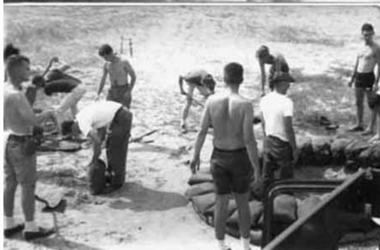
17. Đà Nẵng AB, K-9 Airmen constructing K-9 fighting-holes and bunkers. 1965-1966. Below names agreed upon by Lee Miller, Don Poss, Gary Knutson, and Don Jones.
