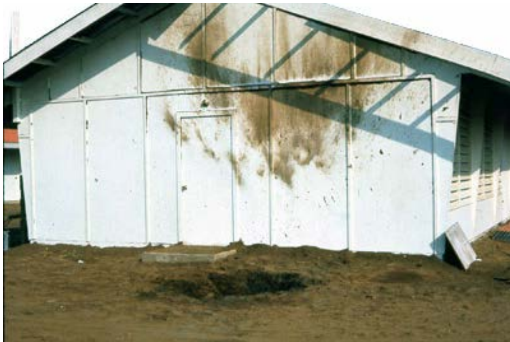
Binh Thuy Air Base, rocket damage. MSgt Summerfield, 1968: 37
