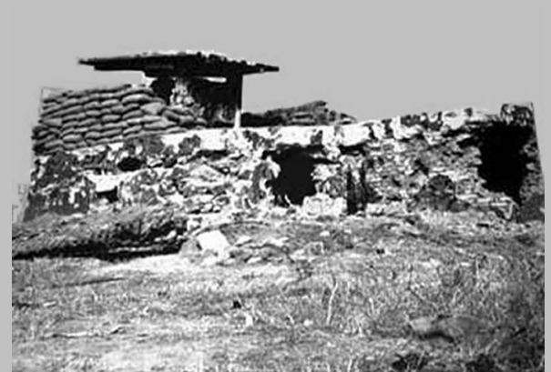
9. Tân Sơn Nhứt AB, Battle damaged O-51 Bunker. Tet 1968. Photo by Steven Shelt, PC 37th; PK, 633rd SPS. 1967-1968.
