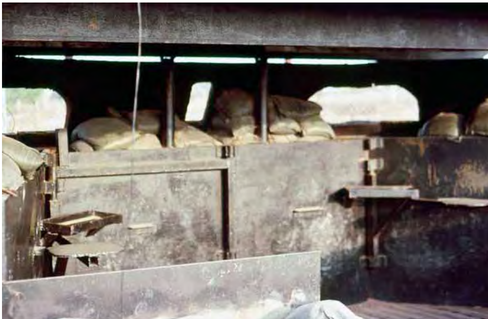
35. Tân Sơn Nhứt AB: Bunker BB7: This is looking inside BB7. They were made of 3/4" steel with a wall like the inside of a house with dirt in the middle. In front of the bunker were sandbags and then 55gal. steel drums. Also there was a cyclone fence surrounding it. this was to prevent mortars hitting the front.
