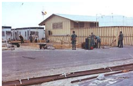
Construction of the warehouse. Notice Vietnamese workers under Air Force guard. Also note watertanks in back of ware house.
