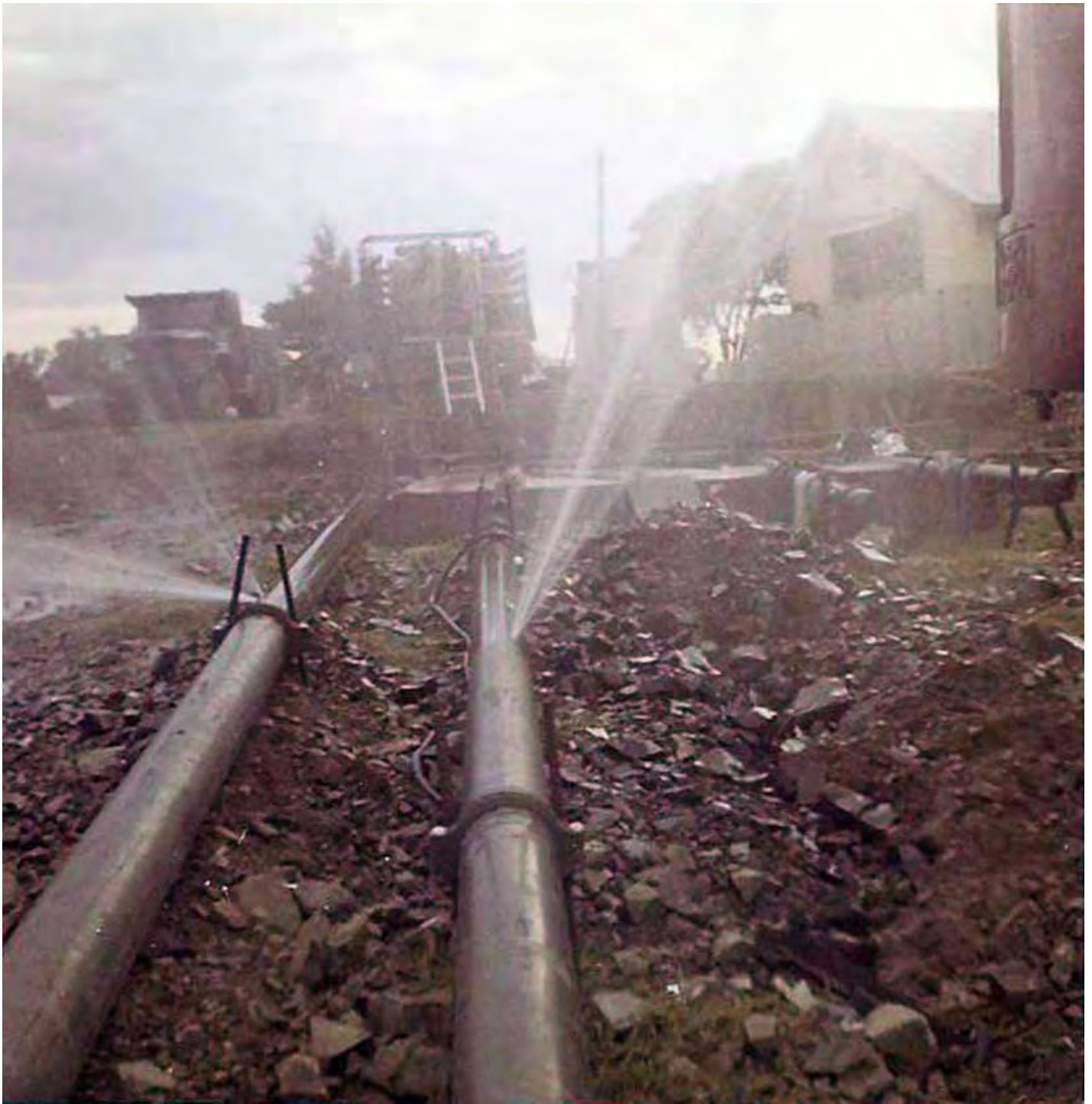
7. Phan Rang AB: Waterpoint Bunker, Outside of Base. Shrapnel punctures in water pipes. Photo by Dana Anthony, 1968-1969.
