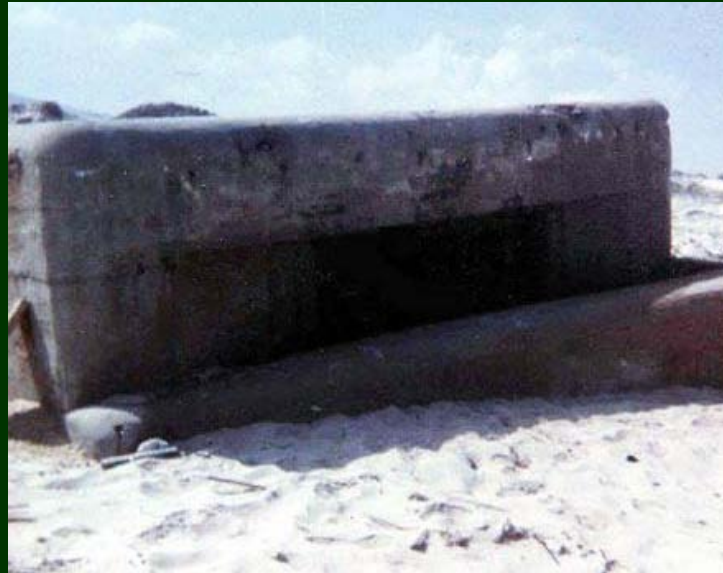
3) Everybody who ever swam on White Beach has to remember this old French concrete pillbox. Cam Ranh Bay AB 1972.
