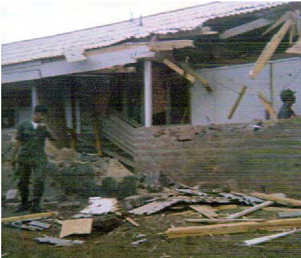
14. Phù Cát AB: Officer Quarters, Rocket Damage. 1970-1971.
