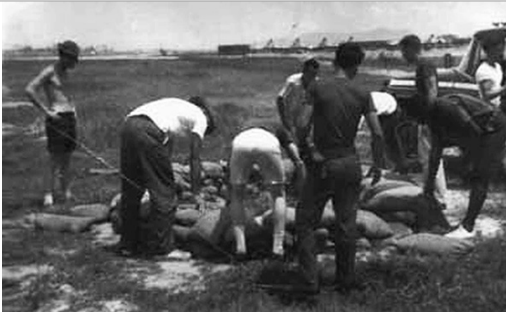
8. Đà Nẵng AB, 366th SPS, K-9: K-9 handlers fortified the first K-9 Fighting Holes between the Active and under construction runways in 1965. Gary Knutson, standing second from right. Don Poss standing with back to camera, fifth from right. Photo by: Lee Miller, 1965-1966.
