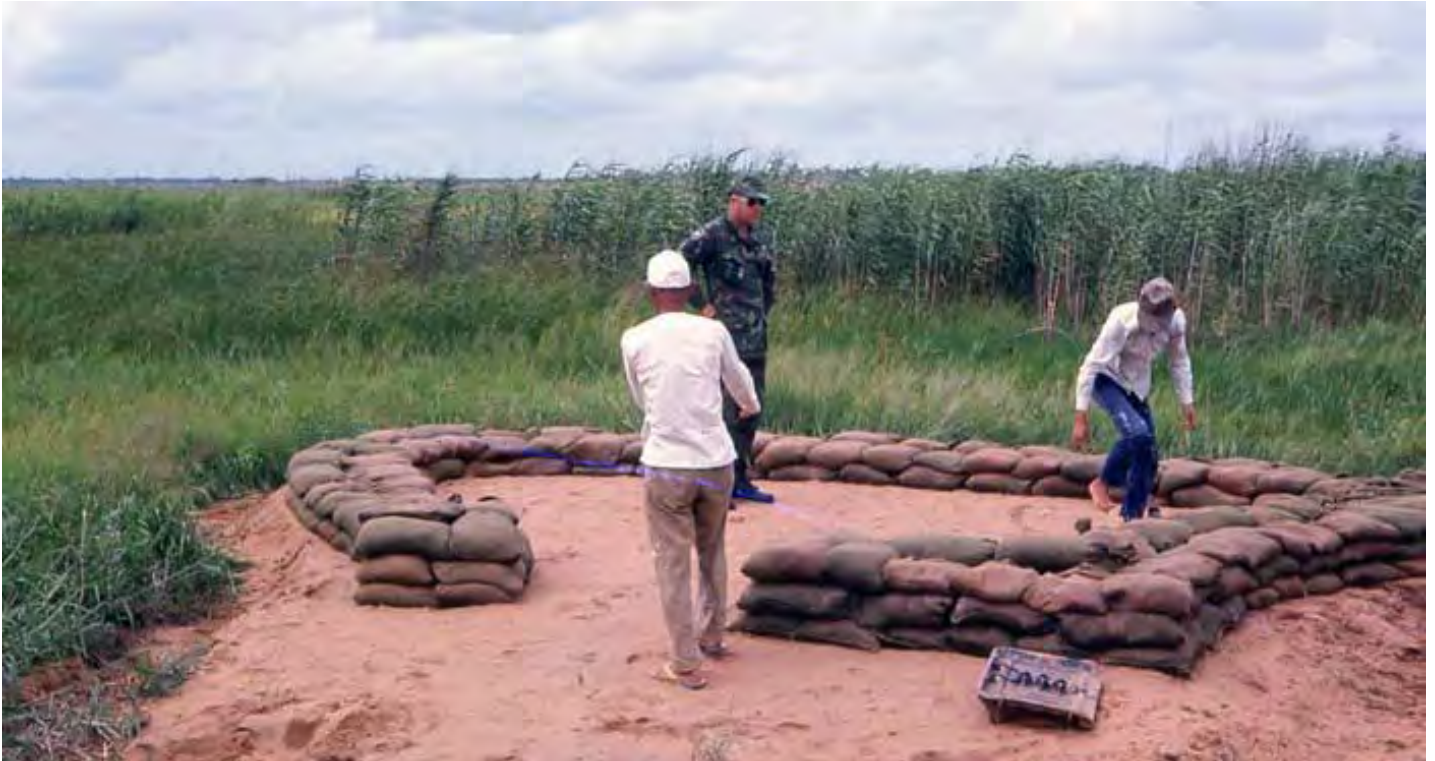
Binh Thuy Air Base, SPS Airman mans instructs Vietnamese workers building Listening Post. M Sgt Summerfield: 07 (Good job... see you tonight! )
