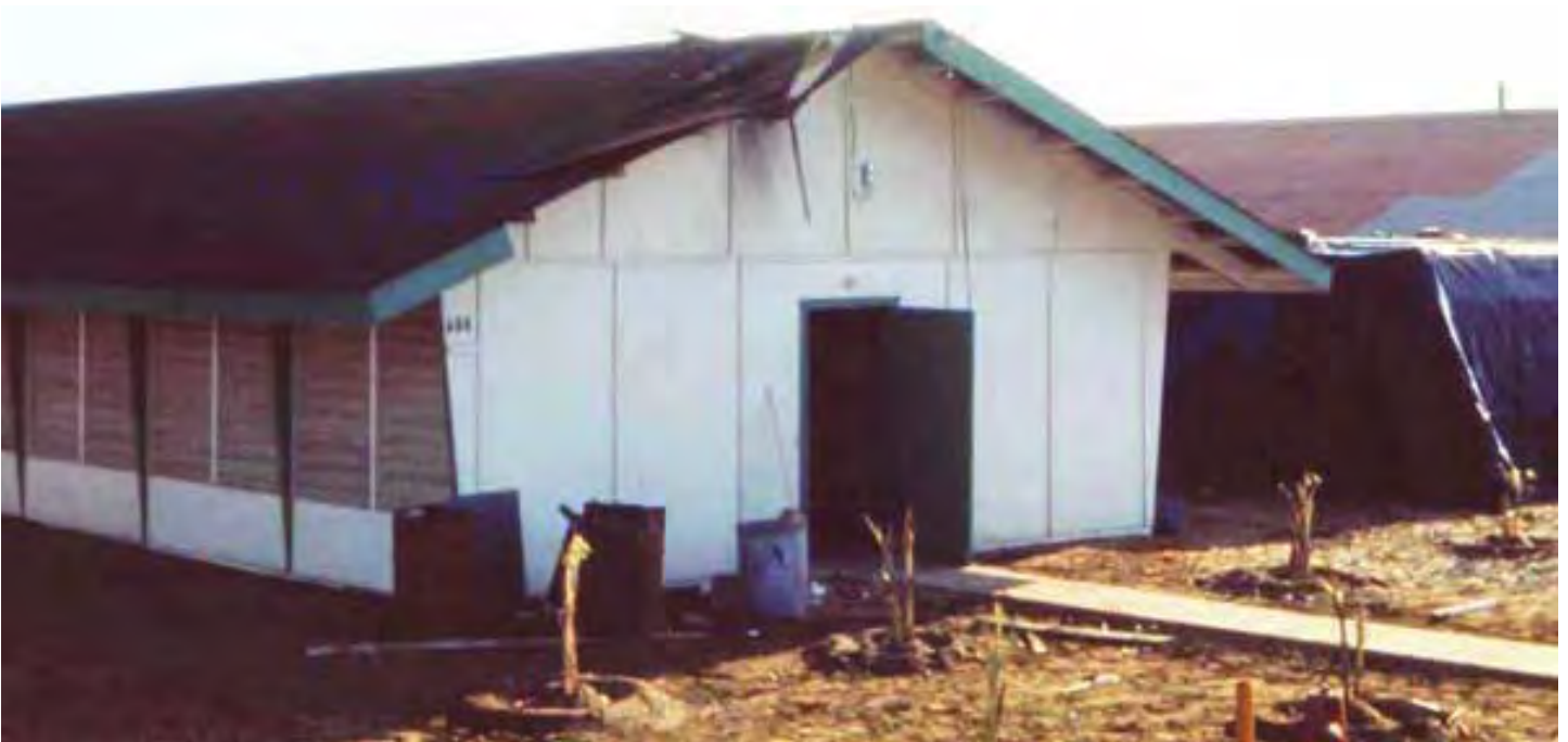
37. Binh Thuy Air Base, rocket damage. MSgt Summerfield, 1968.
