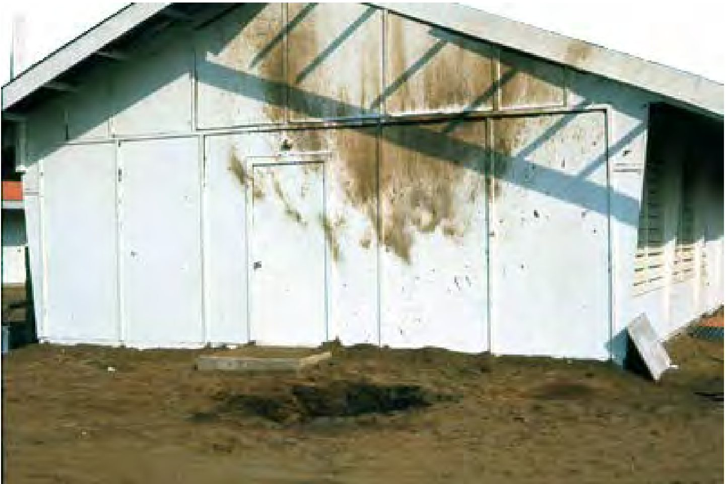
36. Binh Thuy Air Base, rocket damage. MSgt Summerfield, 1968.
